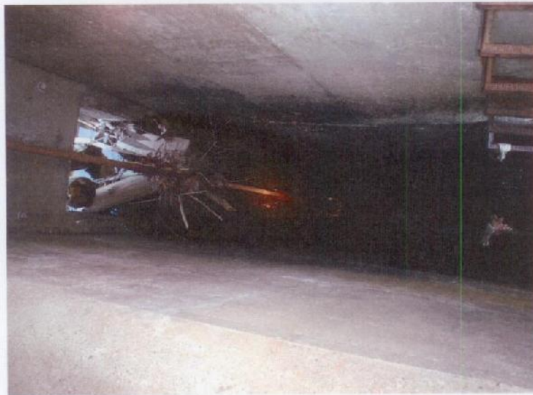
Photograph No. 5: The interior of the principal spillway riser. Note the debris at the low-flow inlet.
