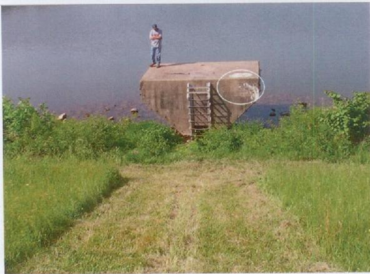
Photograph No. 3: The principal spillway riser. Note the cracking and efflorescence.
