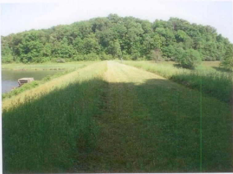
Photograph No. 1: The upstream slope and crest of the dam viewed from the right abutment.
