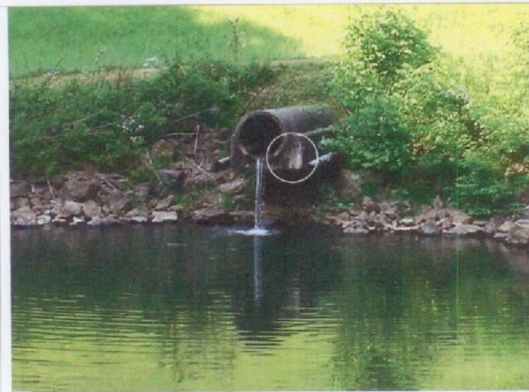
Photograph No. 6: The outlets of the principal spillway pipe and the toe drains. Note the cracks and efflorescence on the concrete cradle.
