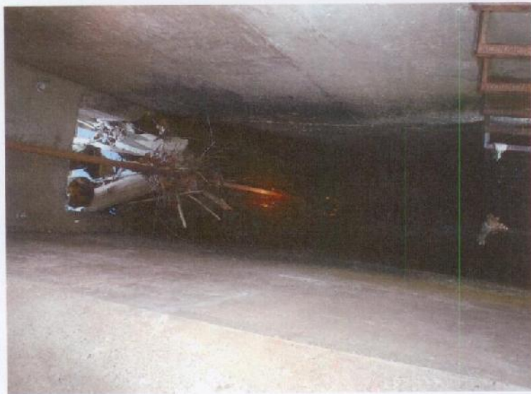
Photograph No. 5: The interior of the principal spillway riser. Note the debris at the low-flow inlet.
