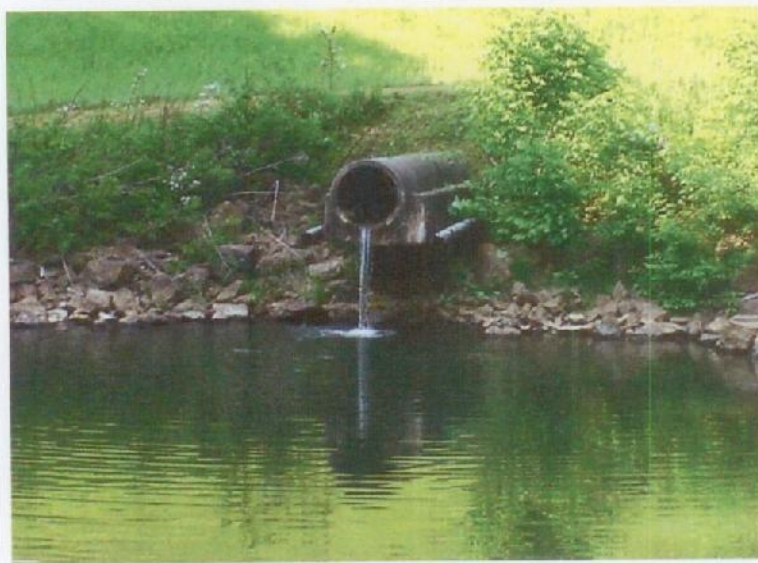
Photograph No. 6: The outlets of the principal spillway pipe and the toe drains.
