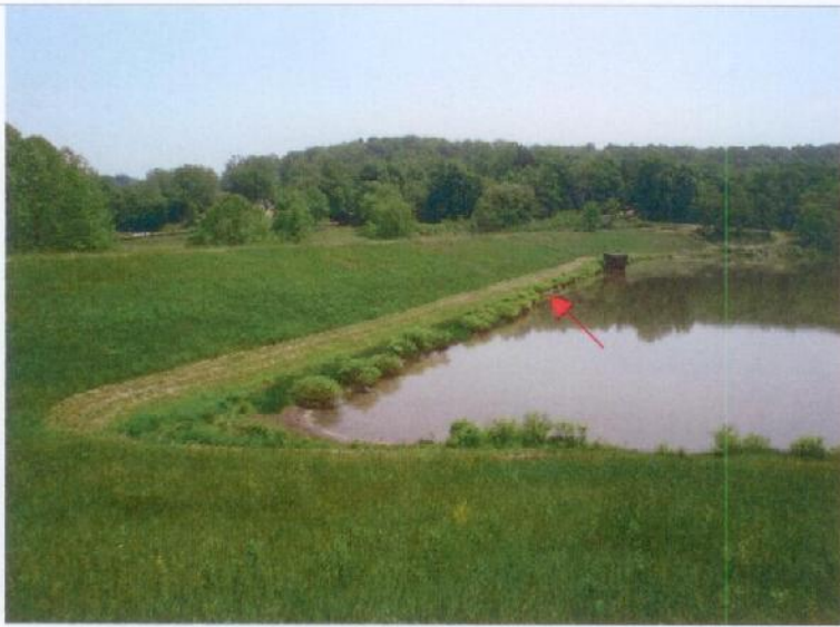
Photograph No. 1: The upstream slope of the dam. Arrow indicates approximate area of minor depression on the slope.
