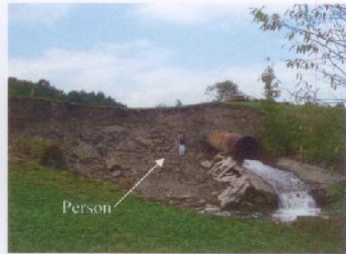
Erosion caused by floodwater overtopping the dam – a result of inadequate discharge/storage capacity and debris obstructing the 5-foot-diameter spillway pipe.
