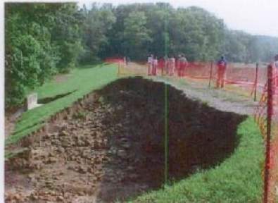
Erosion caused by floodwater overtopping the dam – a result of inadequate discharge/storage capacity.
