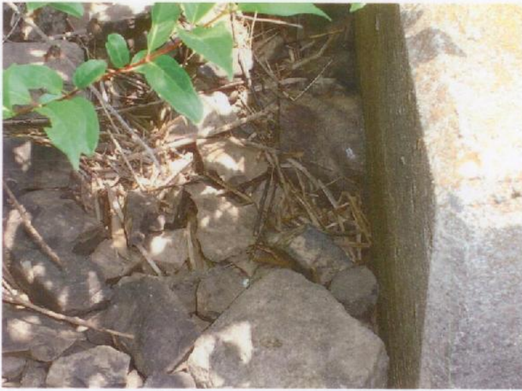
Photograph No. 7: The toe drain outlet. Note the rocks covering the outlet.
