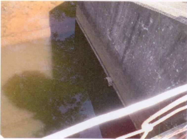
Photograph No. 5: The toe drain outlet on the right side of the impact basin. Note the rusted out invert.
