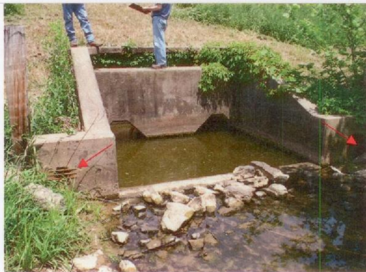
Photograph No. 6: The impact basin at the principal spillway outlet. Note the toe drain outlets.
