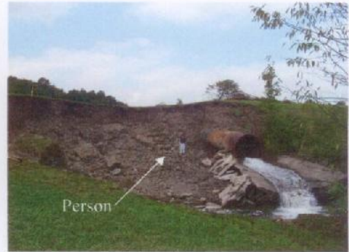
Erosion caused by floodwater overtopping the dam – a result of inadequate discharge/storage capacity and debris obstructing the 5-foot-diameter spillway pipe.
