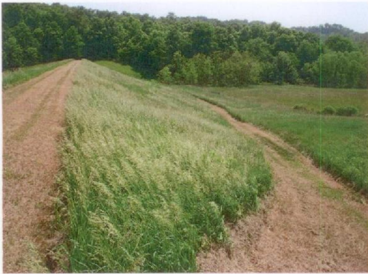
Photograph No. 1: The crest and downstream slope of the dam. Note the tall grass.
