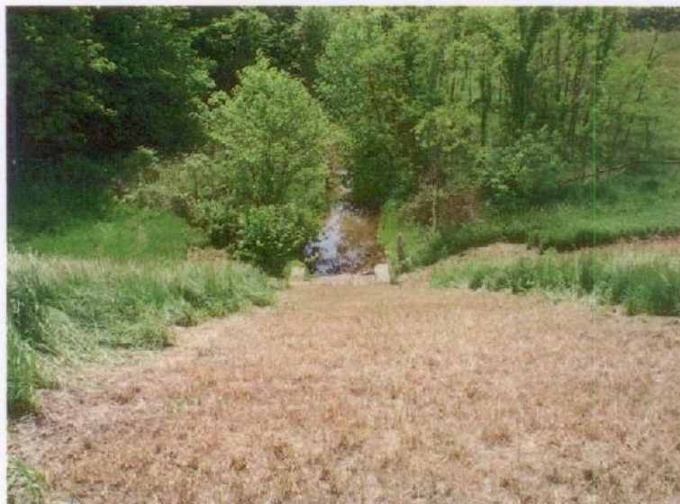
Photograph No. 5: Looking toward the principal spillway outlet from the crest of the dam.
