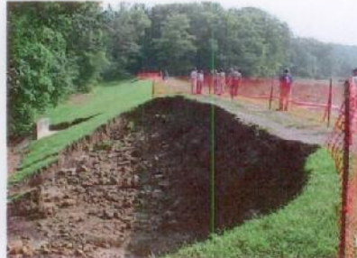
Erosion caused by floodwater overtopping the dam – a result of inadequate discharge/storage capacity.
