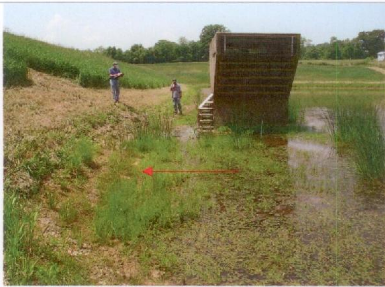
Photograph No. 4: The principal spillway riser. Note the indentation on the upstream slope of the dam.
